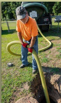
Septic pumping is required every 4 years.
